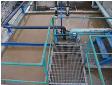
บ่อ Primary Sedimentation tank
