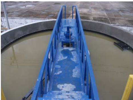
บ่อ Secondary Sedimentation tank
